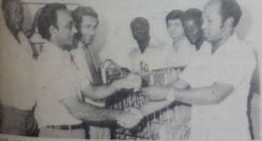
THE Aga Khan Hospital, Mombasa has taken delivery of a new standby generator at its premises on Vanga Road, Mombasa. The generator will supply power to the entire hospital should the mains supply fail. The £15,000 Lister diesel generator's commissioning, supplied by Messrs Machinery Services, marks the second phase of the hospital's five year development plan which commenced this year. The vice-chairman of the Aga Khan Health Service Mombasa Mr Aziz Moya (in glasses) is seen receiving the generator from Hamza the manager of Machinery Services, Mombasa branch. Looking on (from left) are Mr George Mwendo of Machinery Services, Mr Mohamed Mughli of Central Electric House, Mr Jackson, Mr Sadu Dhalila, the hospital administrator and Fred Omondi, the manager of Machinery Services.
