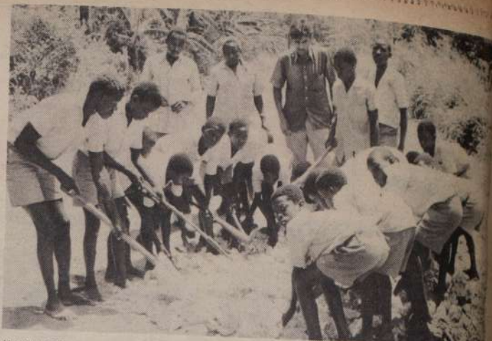
HARAMBEE AT WORK - Supervising the repair of the Utange road is Abid Rajabali, headmaster, Utange Primary School, (third right
