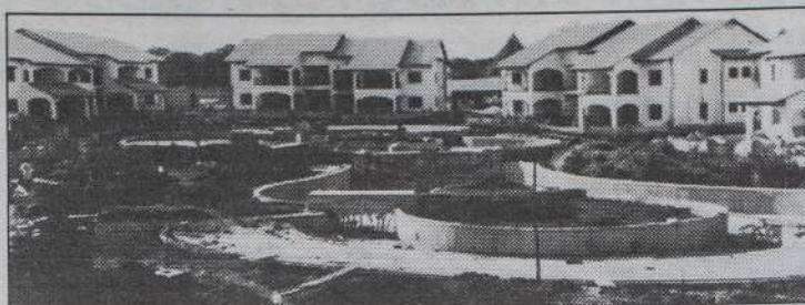
CONSTRUCTION CONTINUES APACE on a unique fresh-water swimming pool at the new Woburn Estate - which will eventually comprise 27 luxury apartments including 14 suites (the largest being 80 sq. metres!) in seven one storage units, the architectural style having a strong Mediterranean influence.
