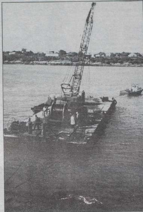
DIVECON Heavy Lift Barge 'Marifa' seen while laying KPLC heavy-duty cables off Mombasa Island.
