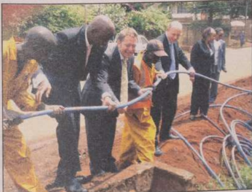
AccessKenya Group Managing Director Jonathan Somen is seen [centre] helping while contractors break ground to dig and lay the new metro fibre optic infrastructure in Mombasa.
