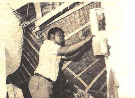
• ENGINEER Khamisi Shungula services an air-conditioning unit at The Banda discotheque - the latest addition to the facilities offered by the Africana Sea Lodge on Diani Beach. The disco premises are fully air-conditioned and have been completed in time for the December holiday season. Each unit is serviced at regular intervals by the hotel staff under the supervision of Mr Shungula. Once a year each air-conditioner is removed and taken to the Car and General workshops on Haile Selassie Road, Mombasa, for a comprehensive service.
