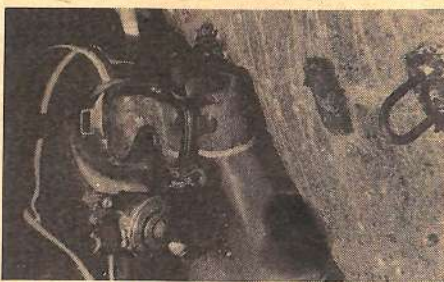
* DIVER/WELDER Hamisi Shai of Divecon is seen underwater welding on the side of the vessel during the early stages of the blanking process.
