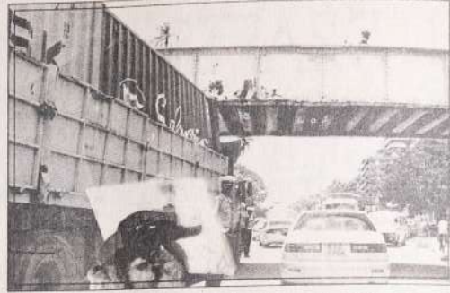
A container lorry is stopped by Police after hitting the Moi Avenue railway bridge near Mombasa's Kilindini Port.
