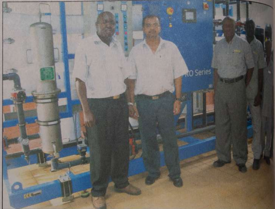
The Serena Group are an important D&S Customer, particularly Mombasa Serena where a D&S supplied Reverse Osmosis Water Treatment Plant treats the brackish well water supply to portable standards. The initial plant was supplied by D&S in 1996 and gave them excellent service over the years though recently reached the end of its life and has recently been replaced by a high tech unit supplied by D&S partner GE Water, specified by Mombasa Mohamed Farook and Operations Manager Daniel Owuor and installed by Technician Kiprono Koech. The Plant recently commissioned and is now supplying 100,000 liters of Pure Water per day to the hotel. The D&S Coast pictured with Serena engineer George Ongaro after the successful installation of the new Serena RO Plant.
