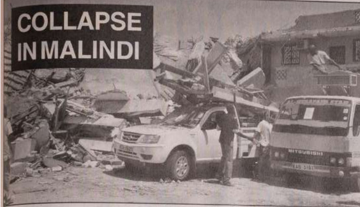
MALINDI (Xinhua) -- Rescuers work at the scene of a collapsed building in Malindi town. One person died and 23 rescued after an eight-storey building which was under construction collapsed on Friday. XINHUA PHOTO - JOY NABUKEWA
