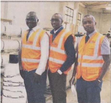
Davis & Shirtliff Mombasa team has successfully delivered and installed one of the largest RO plants ever manufactured by D&S to a local water supply company. 30m/hr Dayliff unit is notable for its 10m long vessels advanced touch screen interface with iDayliff control system. Pictured is the plant during installation with D&S engineers Gilbert Barasa, John Waema and Reuben Masoo.
