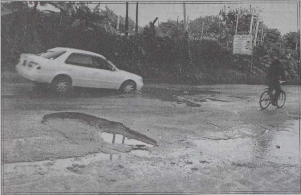
MAYBE THE WORST AREA - This huge pothole, one of several clustered along the main Nyal highway near the Links Road turn off, has effectively turned this major route into a strictly 'one-way' thoroughfare. Long suffering residents despair of any proper repairs to the delapidated section which is obviously made worse by minimal drainage.
