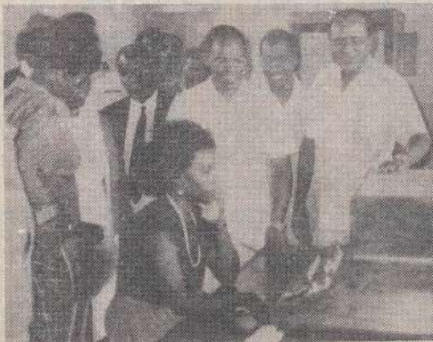
THE TAITA-TAVETA DISTRICT Commissioner Mr P.N. Mbugua tours Manyani manual exchange during the official opening. He is accompanied by the K.P. and T.C. Coast Regional Manager Mr P.N. Mutuku (right), Corporation's Area Manager - Voi Mr Abdi Adan (second right), Chairman Taita-Taveta Mr B. Mvawuganga, other local leaders and senior K.P. and T.C. Regional officials.
